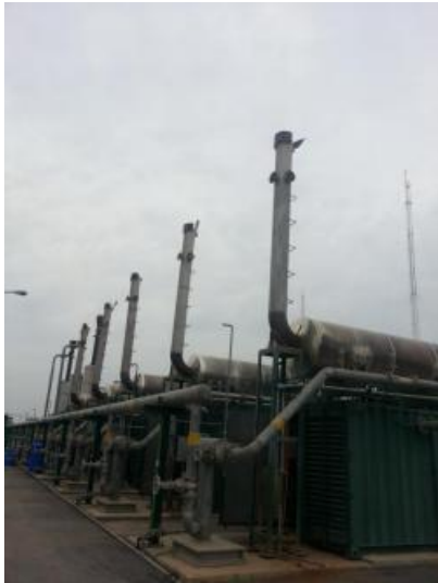
Sindicatum waste-to-electricity generating plant in Nakhon Pathom.
